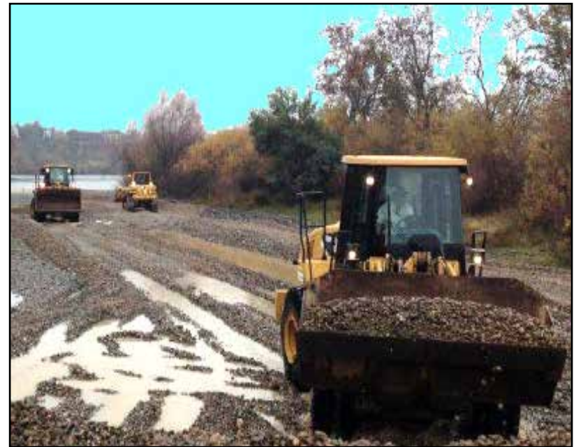
The side channel process levels the area and then covers it with shallow gravel
